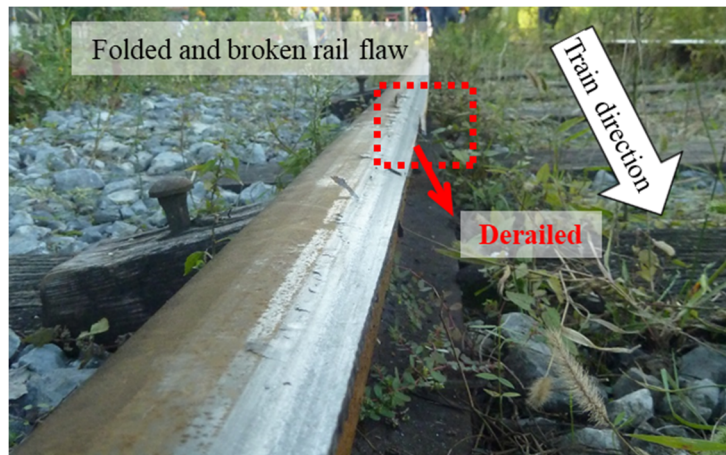
Figure 4. Sample of the derailment to inside gauge as the rail flaw was folded and damaged.
